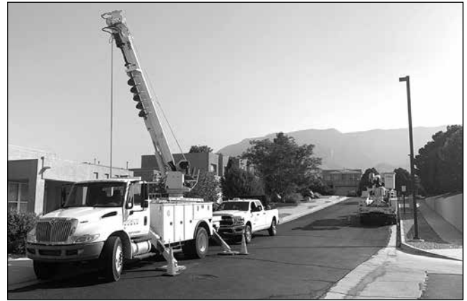
New street lights were installed in Desert Mountain in August by American Power. Neil Wetsch, Director on the Board, provided this photo.
